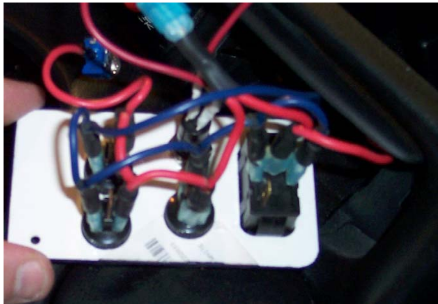
Here is a two stage panel wired using the “Y” technique.
